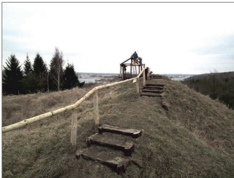
Photograph 85. Construction of a viewing point in the Raduń sub-area (Dolna Odra site) (by P. Pluciński)
